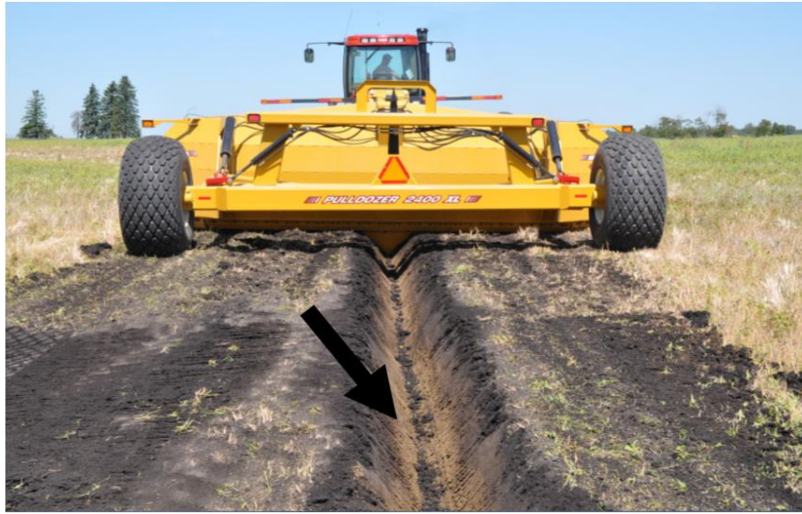
Figure: Trench after the operation with no wind row ridges of dirt left
